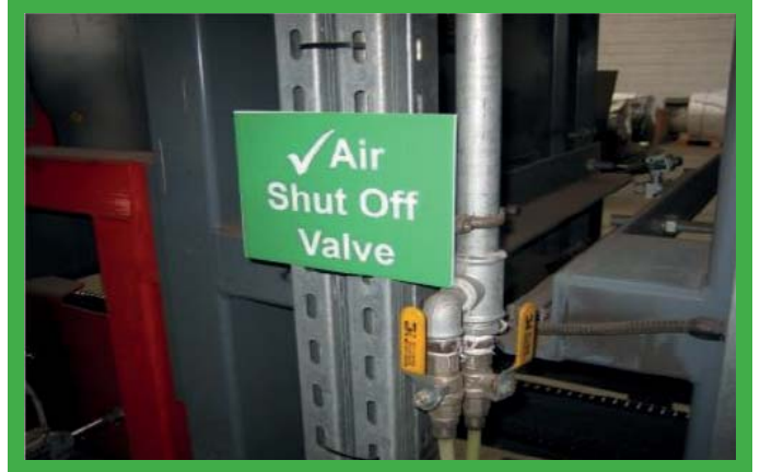
Clearly identified pneumatic isolation point.
