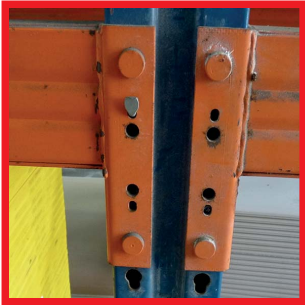
Securing Pins - missing.
