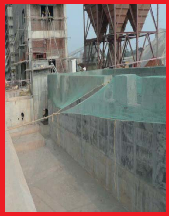
Fatal Accident 2011: Contractor fell while crossing a wall during the construction of an extension.
