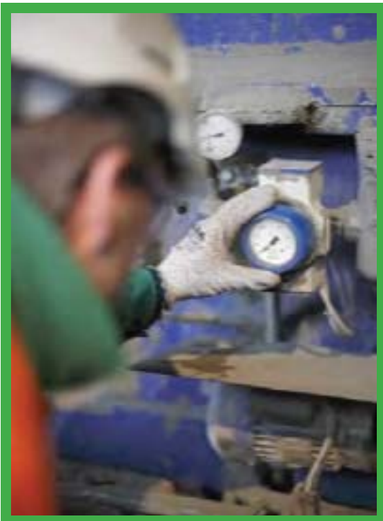
A confirmation check that all residual air has been vented from the system.
