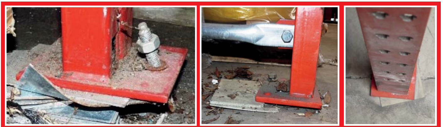
Floor Fixings - broken or missing.
