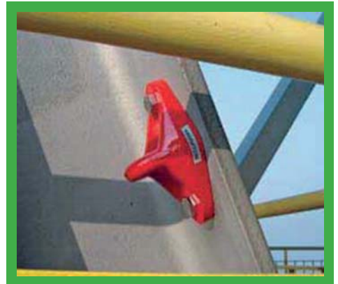
Additional securing hooks for harness use - installed where required.
